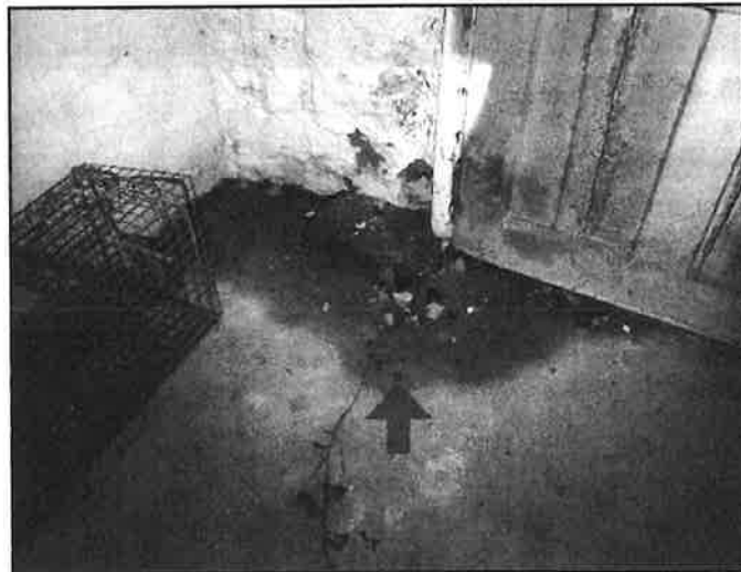
71. Dampness on floor or walls
