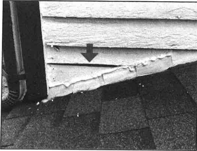
16. Cracked, split or broken
