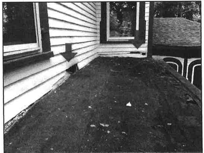
15. Cracked, split or broken
