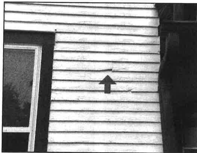
18. Cracked, split or broken
