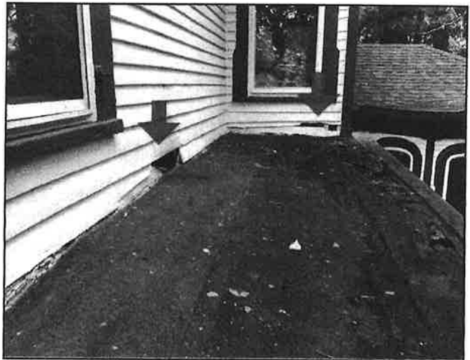
108. Cracked, split or broken
