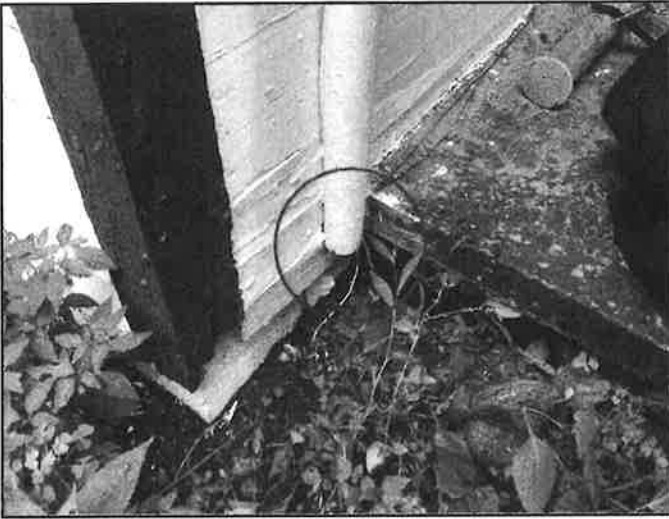
95. Discharge too close to building
