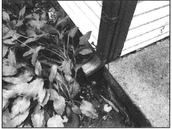
96. Discharge too close to building
