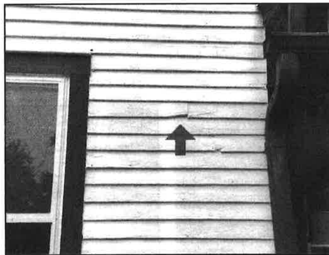
111. Cracked, split or broken
