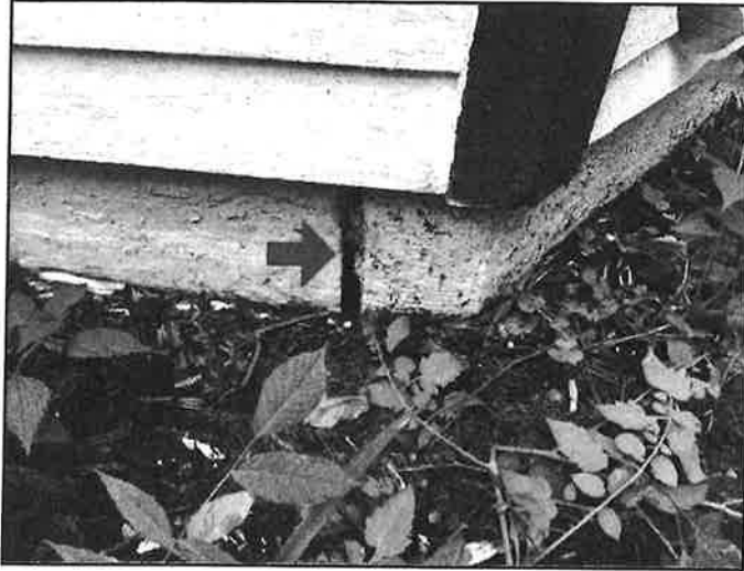
152. Mortar deteriorated or missing
