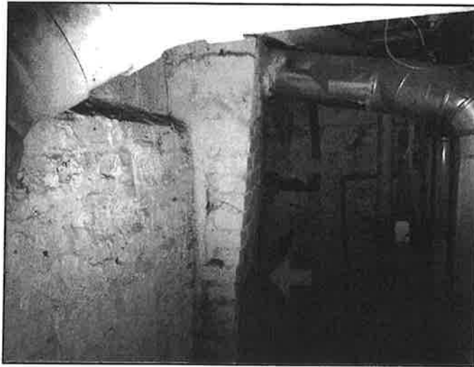
39. Bowed, bulging or leaning
