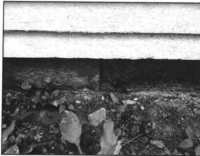
154. Mortar deteriorated or missing
