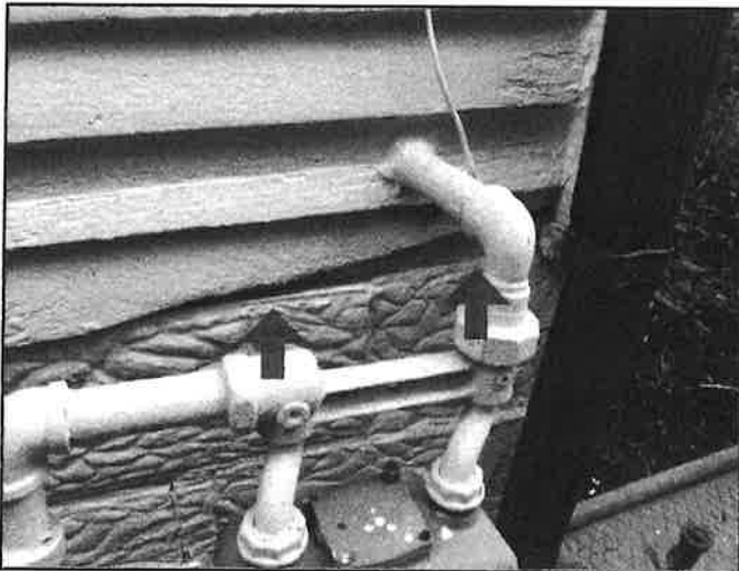
107. Cracked, split or broken
