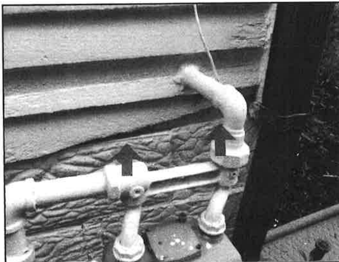
14. Cracked, split or broken
