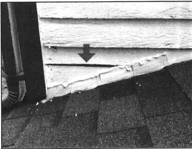
109. Cracked, split or broken
