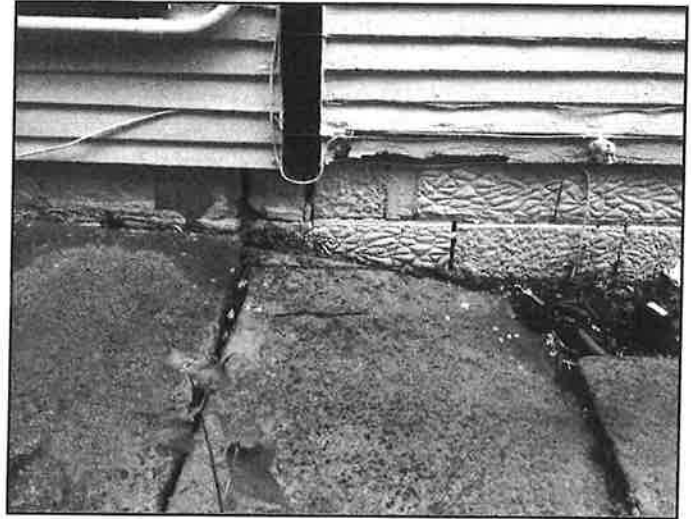
153. Mortar deteriorated or missing
