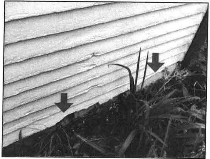
17. Cracked, split or broken
