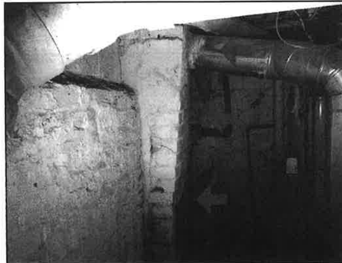
151. Bowed, bulging or leaning
