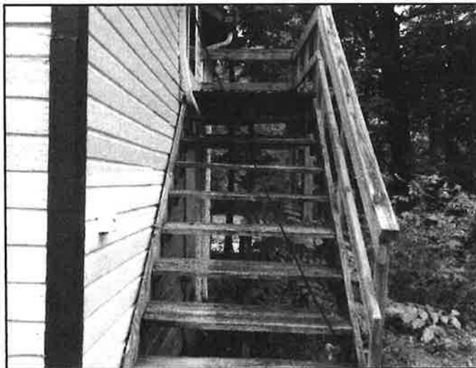
135. Loose Steps / Rot
