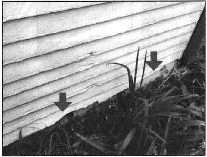
110. Cracked, split or broken
